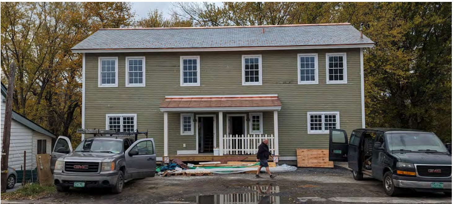
A side-by-side duplex home being renovated in Vergennes, Vermont. Photo Credit: Utile.
