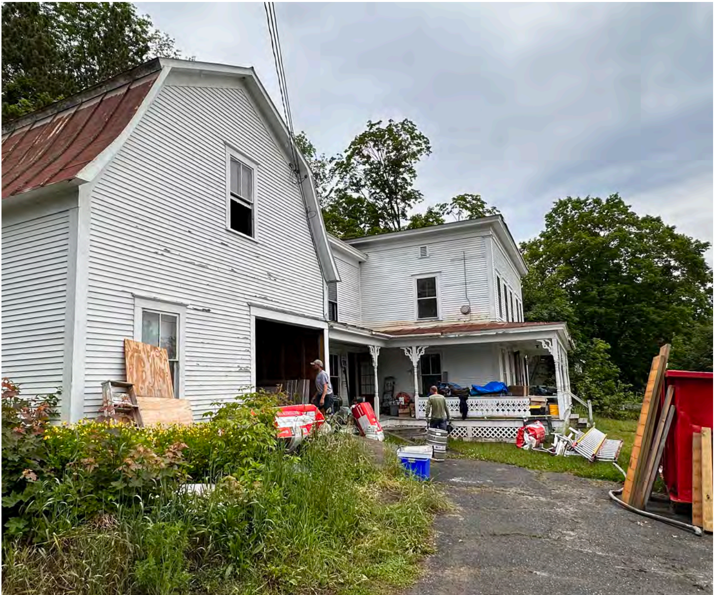
Renovations underway at small-scale developer Jonah Richard's project in Bradford, Vermont. This rehab project takes advantage of the configuration of this vernacular connected farm building to create a multi-unit development from what was once a single unit farmhouse and barn. Photo Credit: Jonah Richard.
