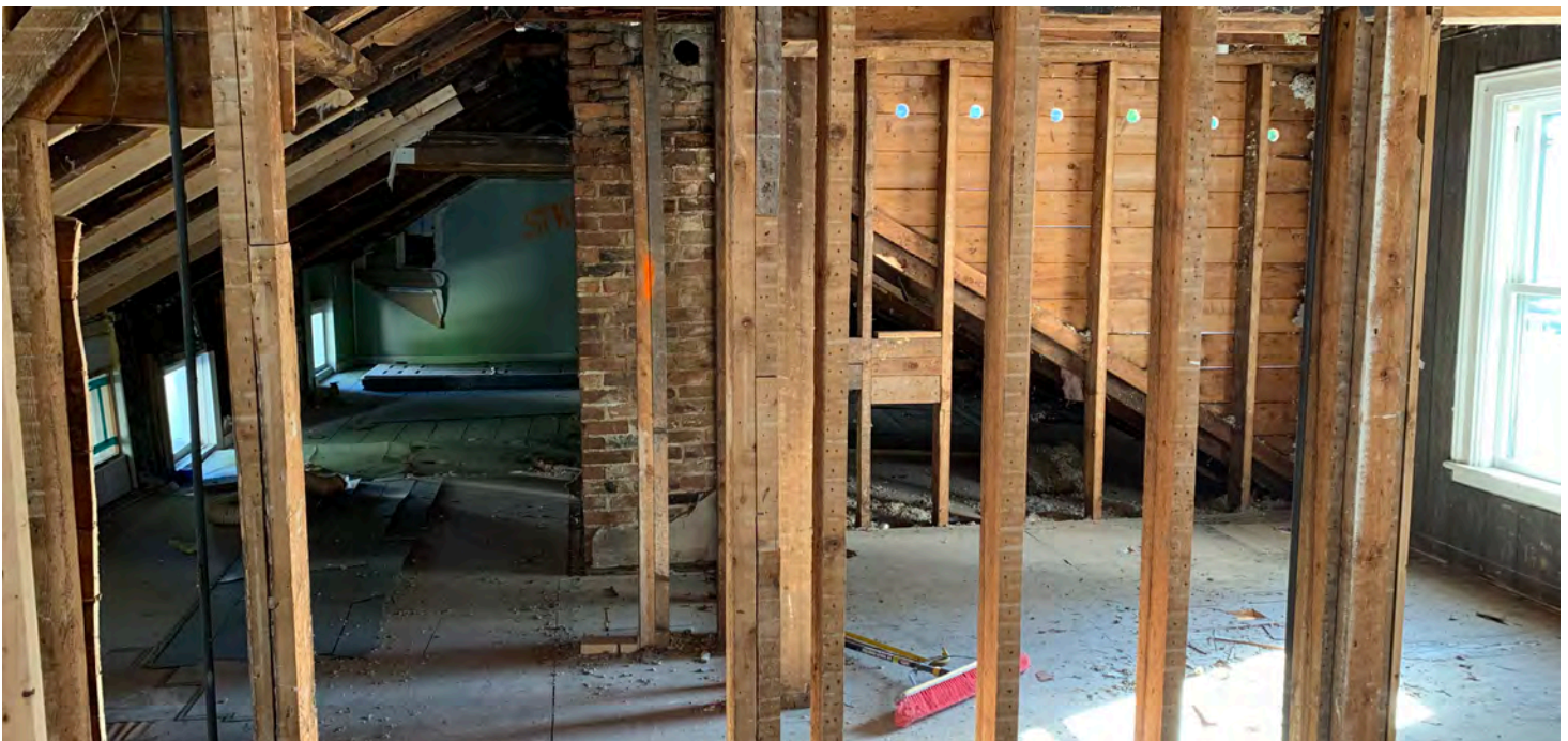
Exposed studs in the attic during a gut rehab and conversion of a historic home by small scale developer Zak Hale of Hale Resources in Bennington, Vermont. Photo Credit: Zak Hale.
