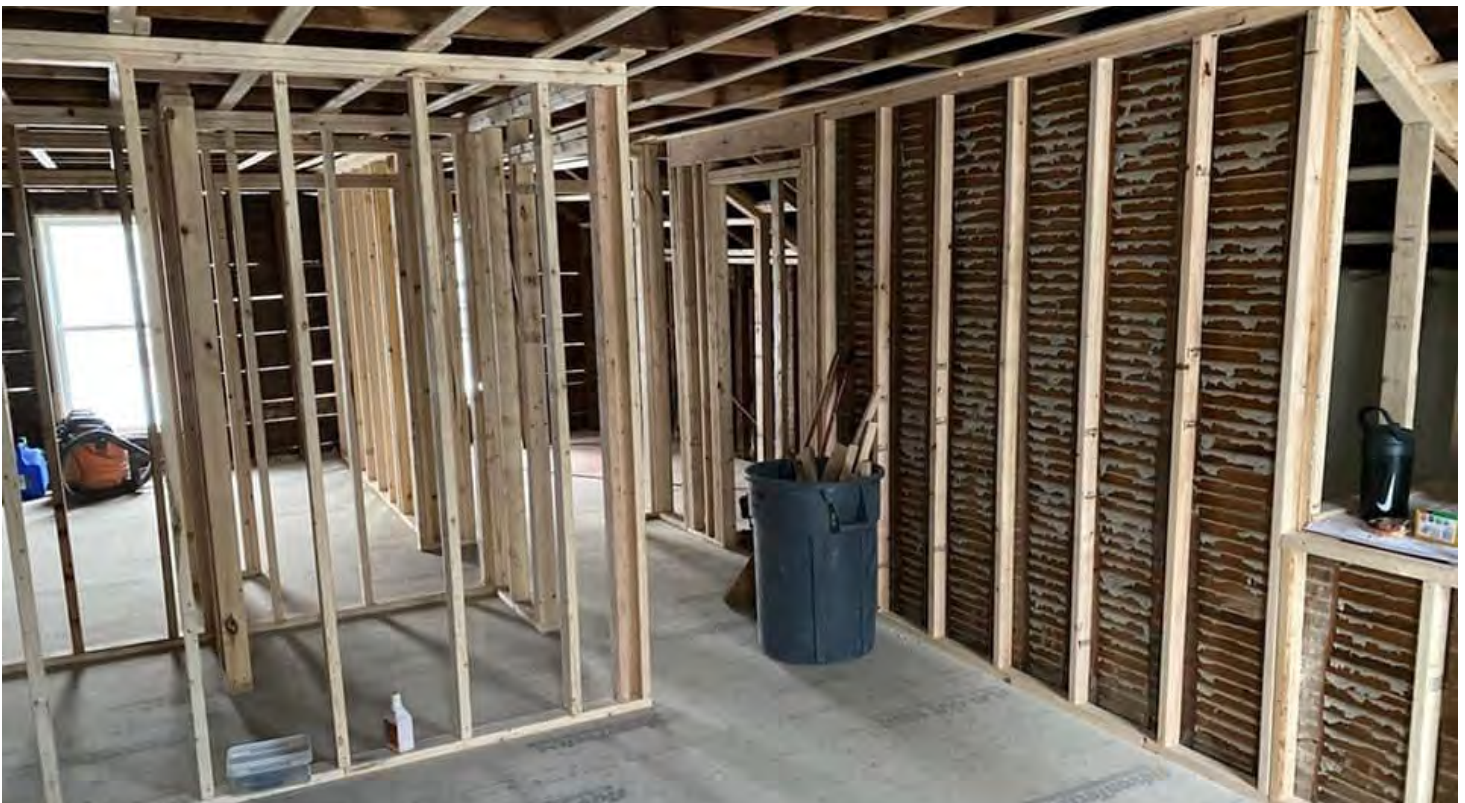
Exposed studs during a gut rehab and conversion of a historic home by small scale developer Zak Hale of Hale Resources in Bennington, Vermont. Photo Credit: Zak Hale.
