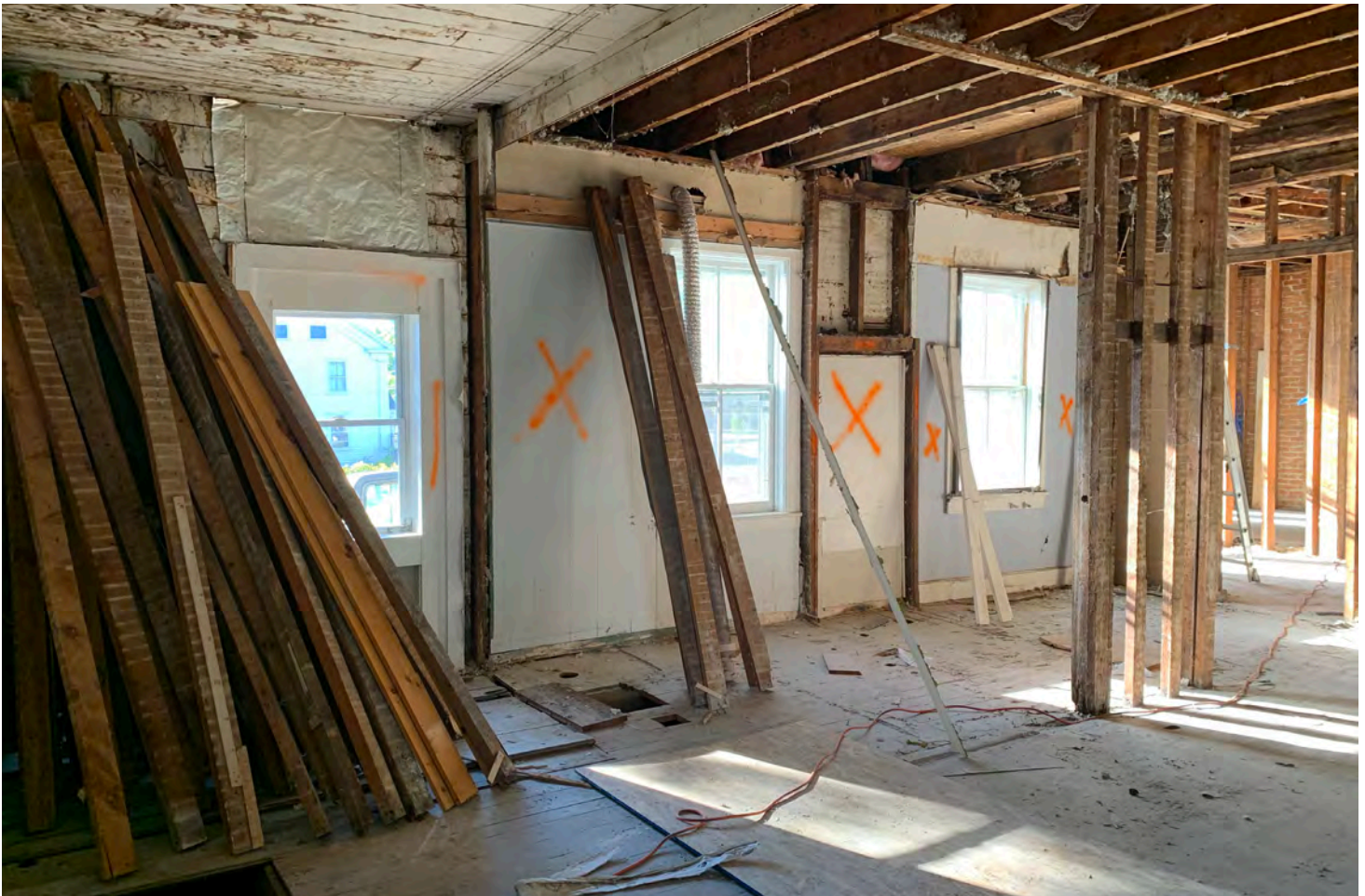
Construction in progress at one of small scale developer Zak Hale of Hale Resources' renovation properties. Photo Credit: Zak Hale.
