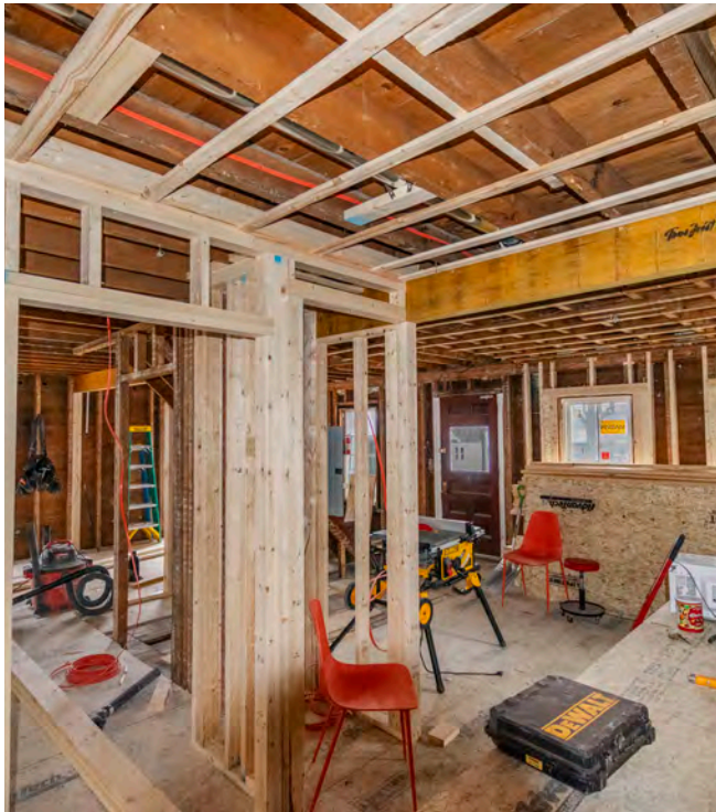
Construction underway at Jonah Richard's renovation of a historic home in Bradford, Vermont.
